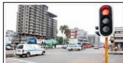
Figure 1.62 - Traffic Lights Control System
